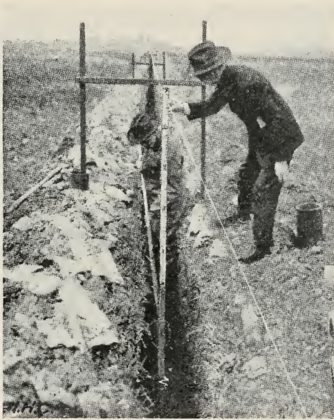
Fig. 11.—Measuring down from an overhead cord to make sure that the completed trench is everywhere seven feet from the line. (Courtesy of International Harvester Co.)
